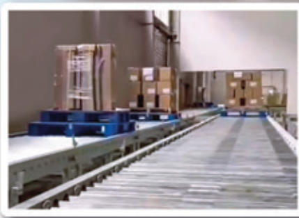
連廊智能運輸系統 Intelligent Transportation Systems
